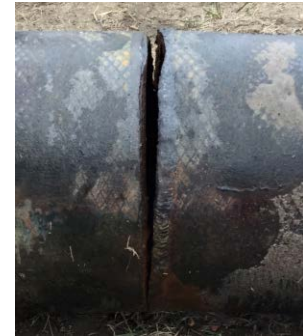
Close-up of the breach in the Poplar Pipeline, after the section had been excavated in April 2015 (source: Bridger Pipeline LLC)
