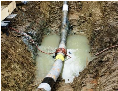
Repair clamp (in red) on ruptured section of the line, pending replacement of the section (source: wvxu.org)
