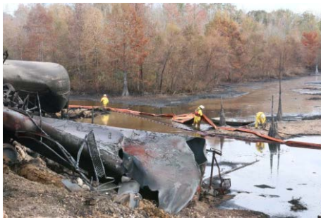
Containment and recovery on a marshy site: laying containment booms next to the damaged tanks (Source: US EPA)
