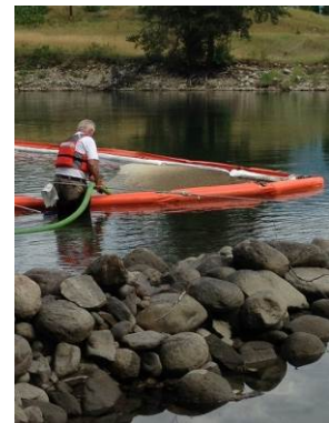
Containment by floating and sorbent booms and recovery by pumping (vacuum truck) (Source: Lemoncreekresponse.ca)
