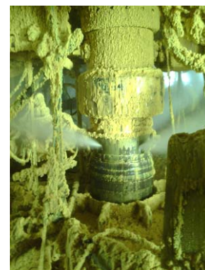
The Elgin G4 wellhead: view of the source of the leak (Source: Total)
