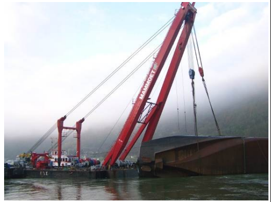
Stabilising the barge Waldhof using sheerlegs during salvage operations (source: Mammoet Salvage)
