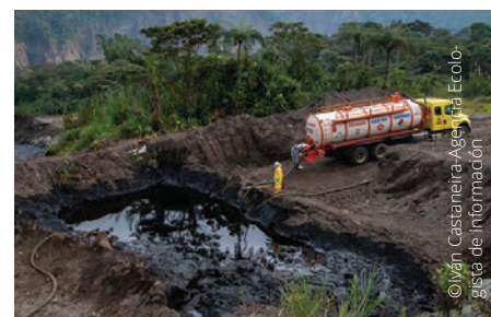
^ Crude oil containment/collection using sorbent booms in secondary drainage pits along the ravine (top); pumping (vacuum truck) to a collection point/pit (bottom).
