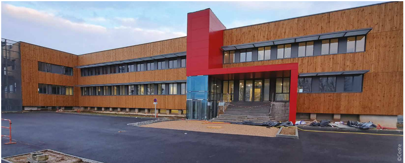
^ Finistère fire and rescue service's new training centre under construction in Saint-Ségal, Brittany
