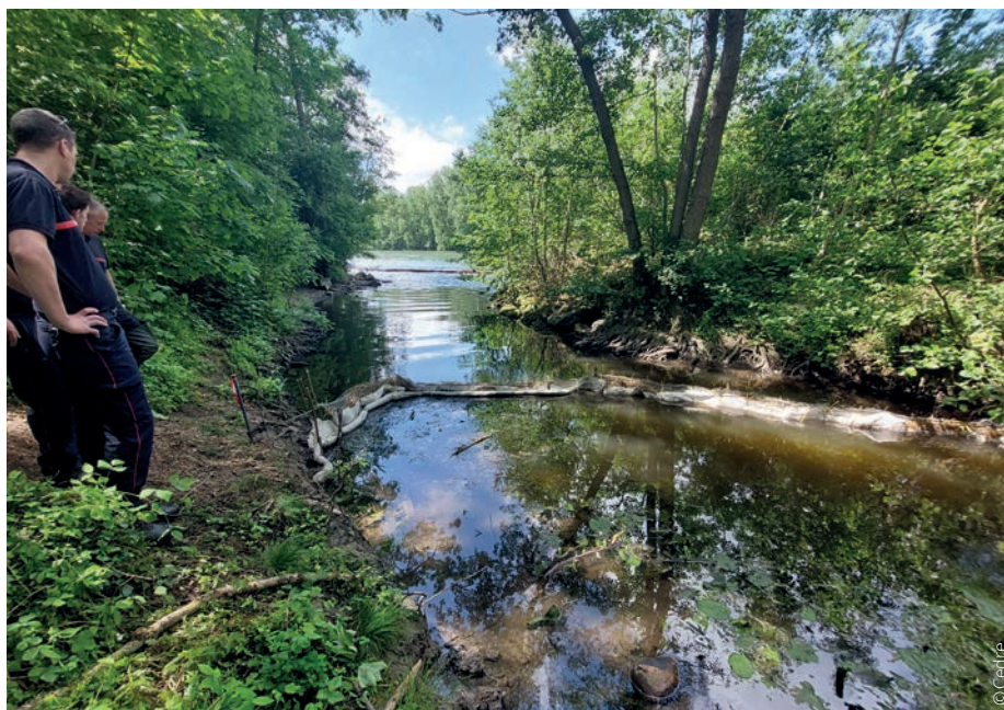
▲ Custom-made barrier (wire mesh/straw) built by the Val-d'Oise fire brigade upstream of the confluence with the Oise
