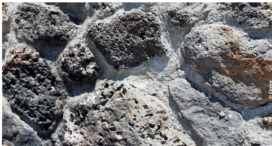
▲ Checking for any oil that may be remobilised or likely to cause oiling due to rubbing, present on the surface or in the cracks/pores of a port structure (here: grouted stone wall treated by rinsing followed by high-pressure cleaning)
