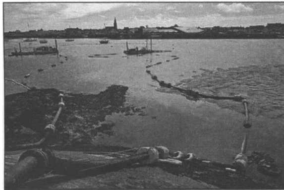
Figure 6. Overall view of the dredging system: two suction dredges anchored on piles and the hoses that deliver the polluted sand and water to the settling lagoon.
