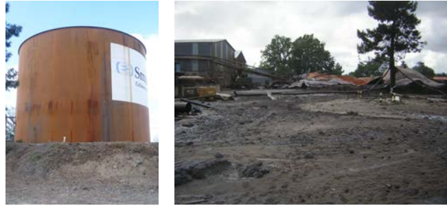
Black liquor tank, before (left) and after (right) its rupture on 5th July 2012 (Source: DREAL Aquitaine)
